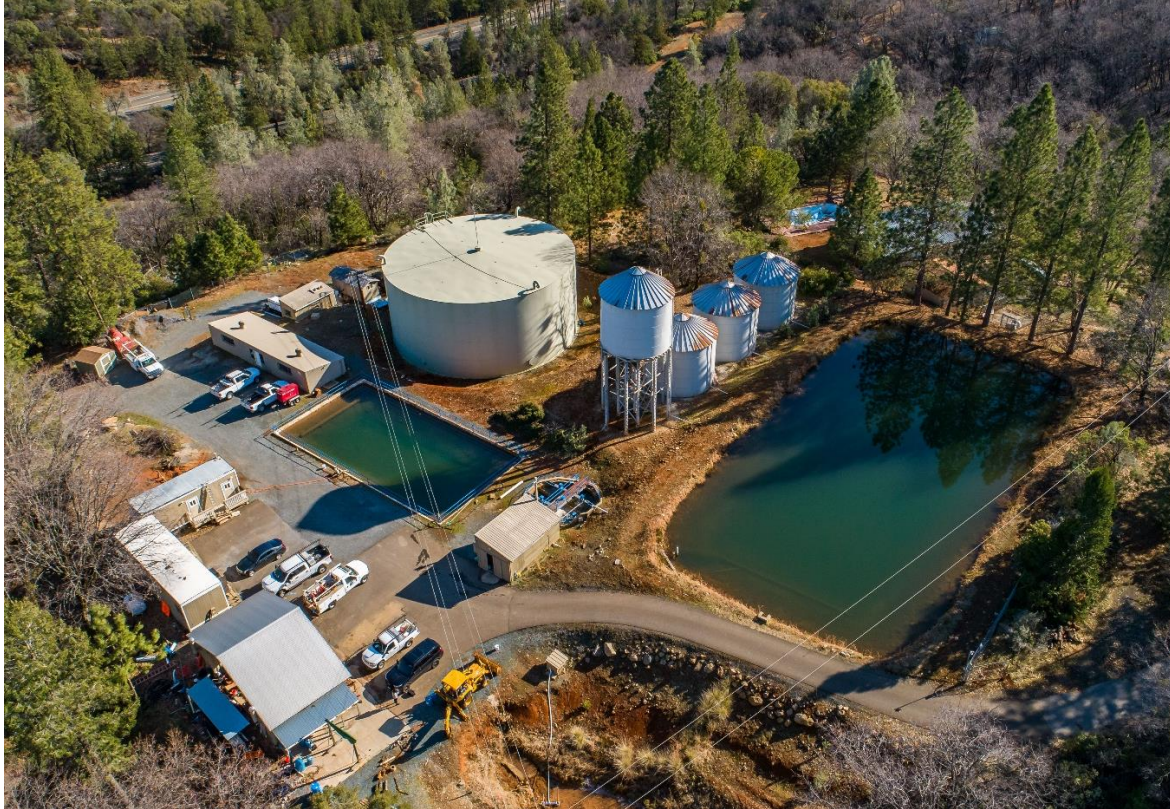
A view from above of the Weimar Water Company water treatment plant facility.
