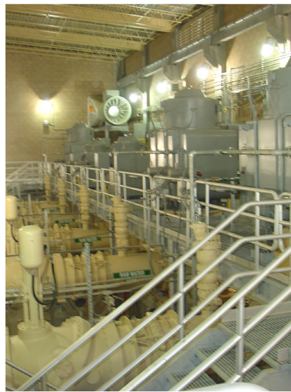
Pump Station The 2-level pump station was constructed partially below-grade to follow suit with other non-invasive project elements.
