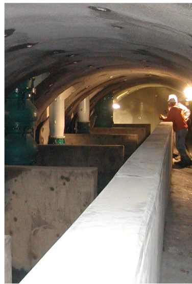
Vertical Pump Shafts Seven 54-inch diameter vertical pump shafts were drilled approximately 75-feet into bedrock to set the pumps.
