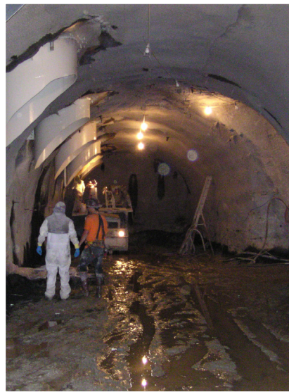
Pumping Well The pumping well was tunneled into bedrock 90-feet below the pump station and hidden from public view in the canyon wall.
